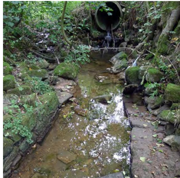
Footbridge over Coundon Burn, collapsed - Auckland Castle Park
